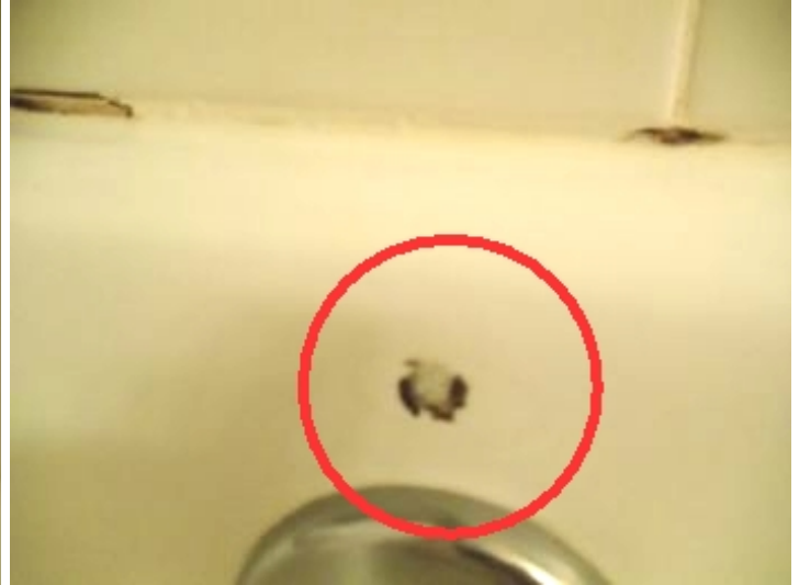
Damaged porcelain finish of tub
