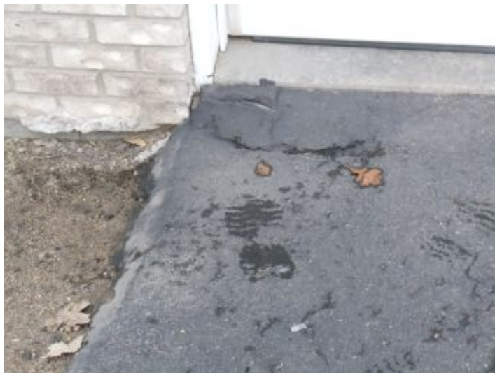
Settling in front of garage and along house
