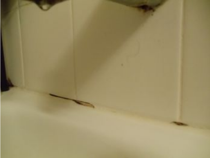
Deteriorated caulking with mildew formation around tub
