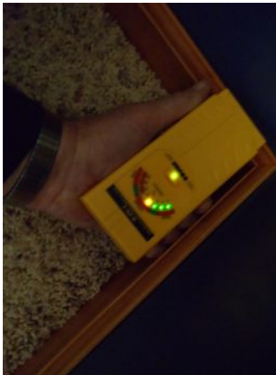
14% moisture reading taken in southwest corner of room.
