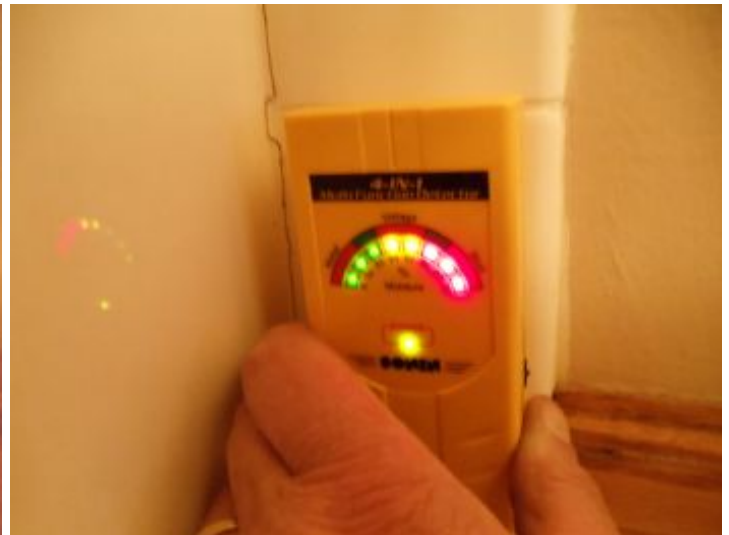
High moisture reading in corner next to tub. Recommend watching this area for mold and mildew growth
