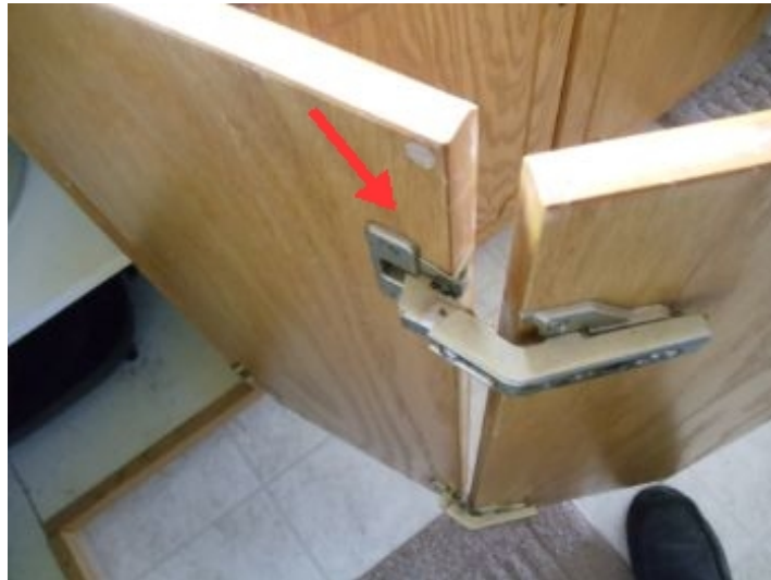
Corner cabinet hardware loose
