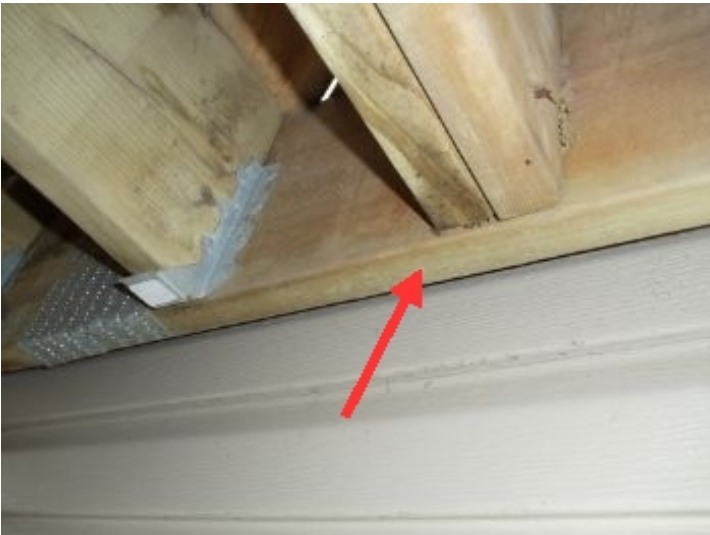
Joist hangers missing on some joist
