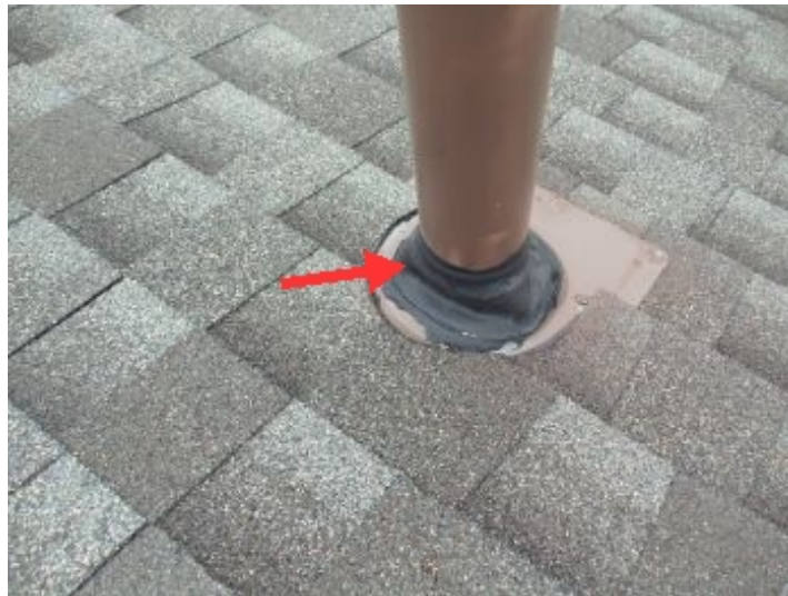
Pipe sealing cap needs caulking
