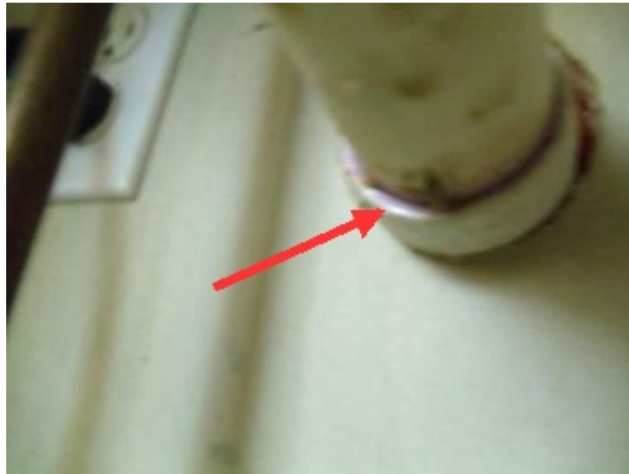
Evident leak build up to main drain piping
