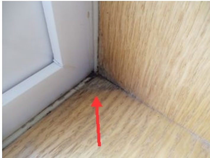
Moisture damage to window sills
