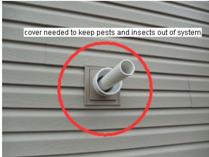
Exterior vent cap combination missing
