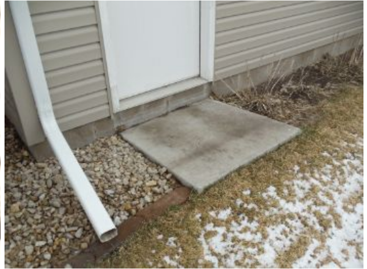
Slab for garage door settled and tipping toward garage
