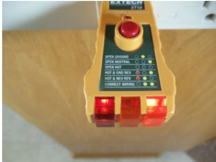
Outlet on island reversed hot and neutral
