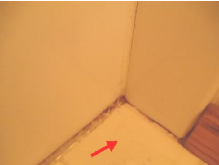
Evidence of moisture damage to floor
