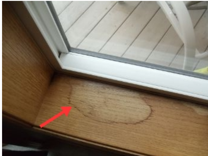
Windows show signs of moisture damage from window condensation in winter
