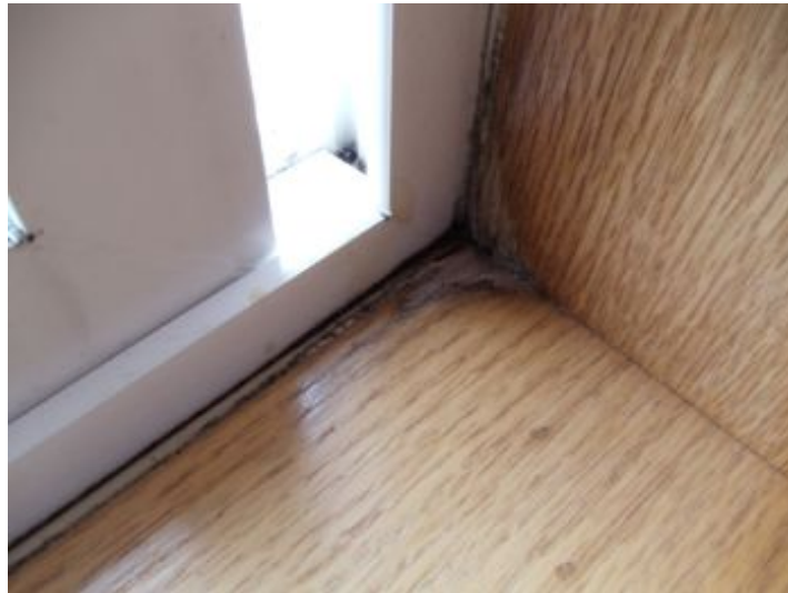
Moisture staining at bottom of front window
