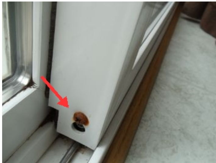
Rusting screws indicating moisture condensation in winter
