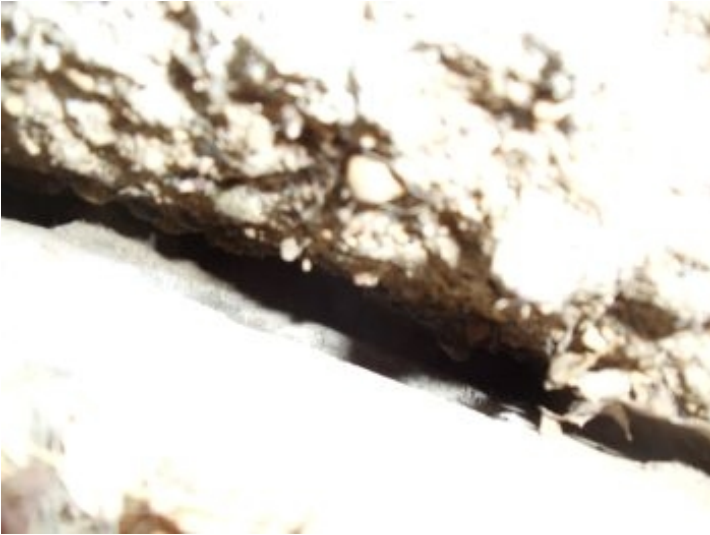
Front stoop slab not sitting on foundation
