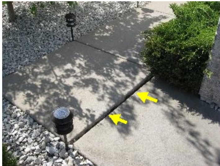
Grounds Sidewalks condition
